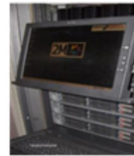
Hardware and Software (HMS solution) Installation and configuration
